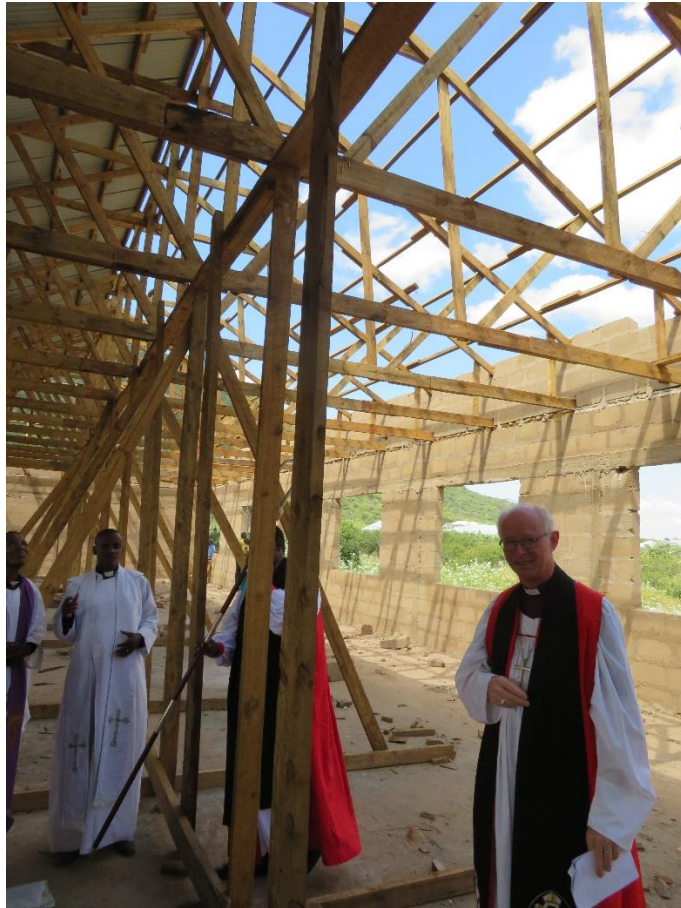
Bishop James of Rochester UK laying the Foundation Stone for the Dining/Assembly Hall in May 2018
