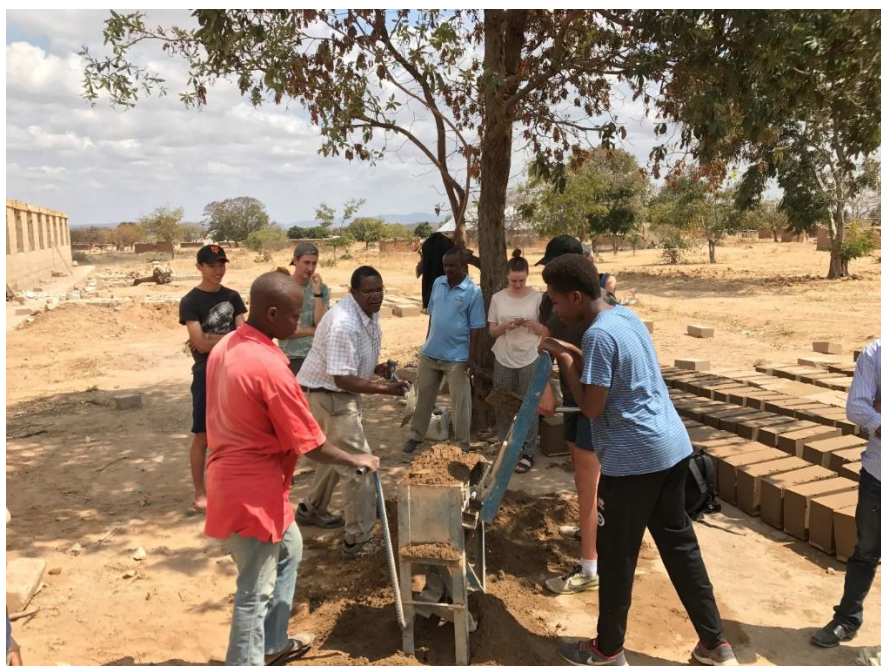
Bishop Given and his son Amani making bricks at the Chemba Secondary School site with the young people from St Peter & St Paul in August 2017
